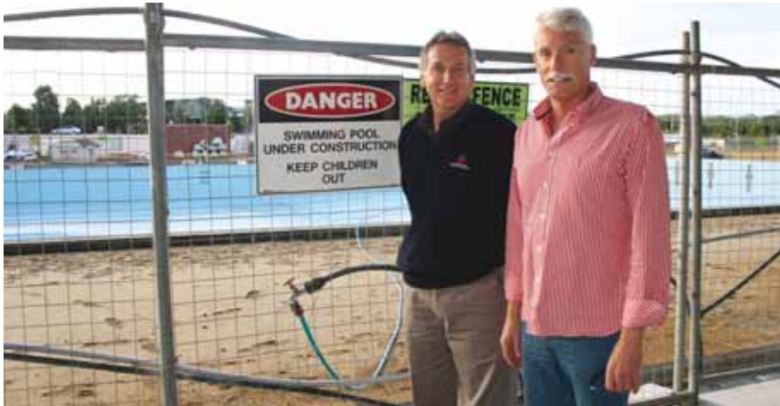
■ Professor Brendan Burkett and Phil Hubble inspect the progress of USC's swimming pool.
